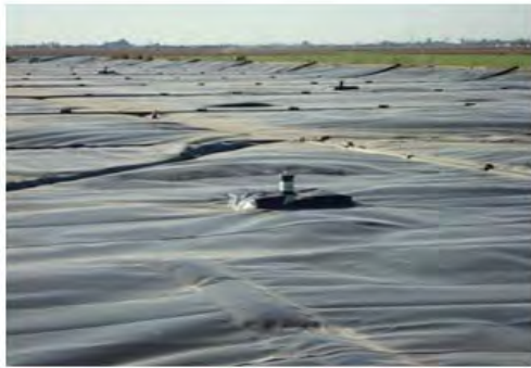
Covered Lagoon Digester
