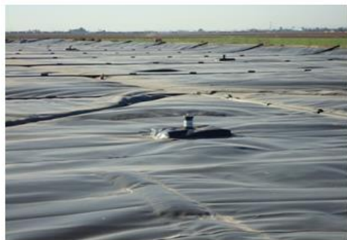
Covered Lagoon Digester
